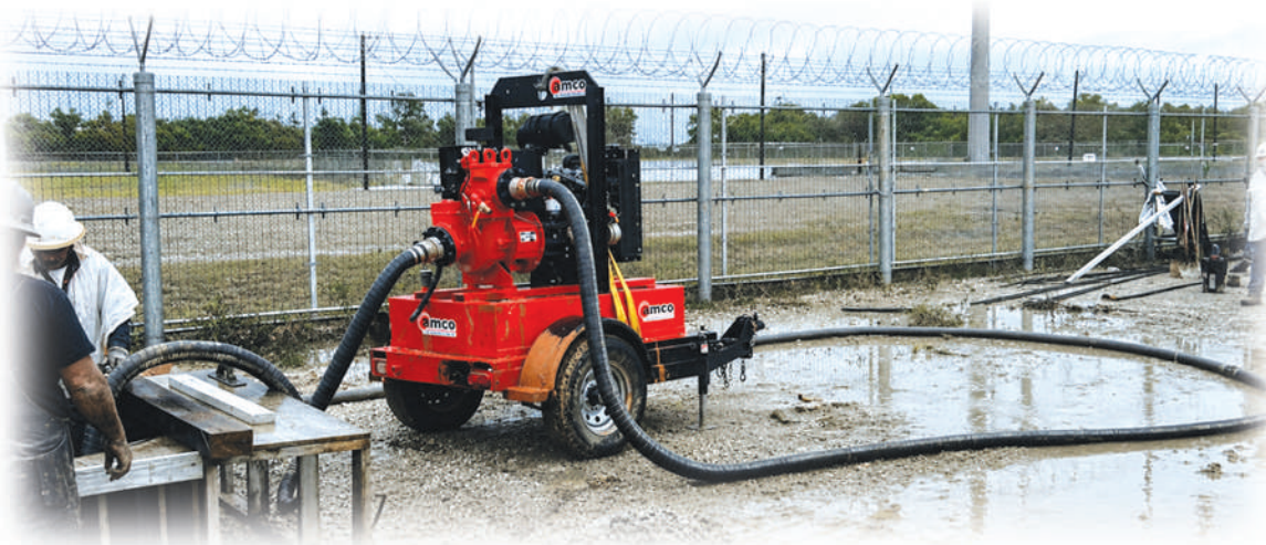
AMCO Pump in operation
